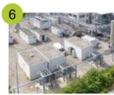
Grid injection plant
