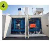
Liquefier and e-LNG filling station
